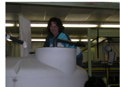
2004/2005 - Girdwood Wastewater Treatment Facility Membrane Bioreactor (MBR) Pilot Plant Project – WE engineers were the operators! From installation thru monitoring AND cleaning up all messes!
