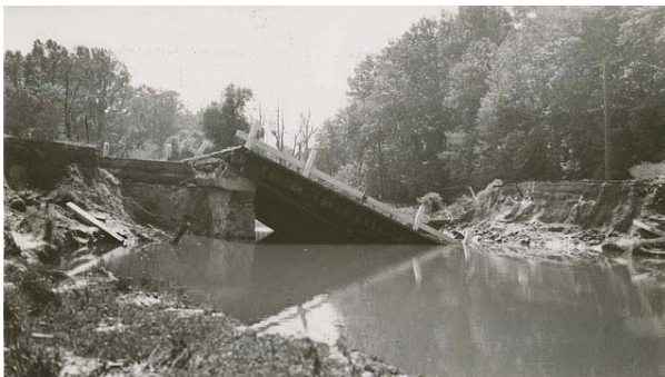
Damage to the Jefferson Bridge over Edwards Run Millville, New Jersey
