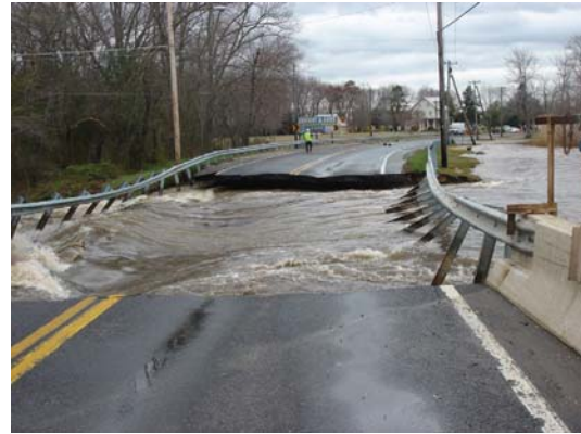
Rainbow Lake Dam Failure – April 15, 2007 Pittsgrove (Salem County), New Jersey
