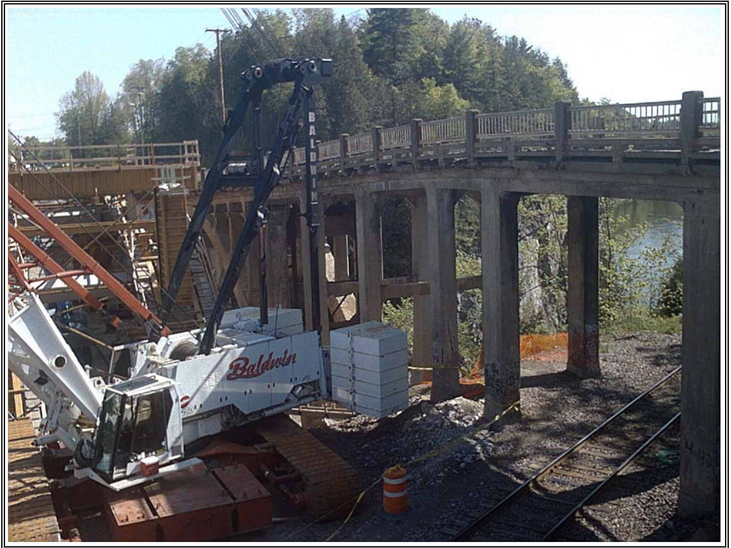
View of the old bridge and construction of the new Lime Kiln Bridge (as of 5/24/06).
