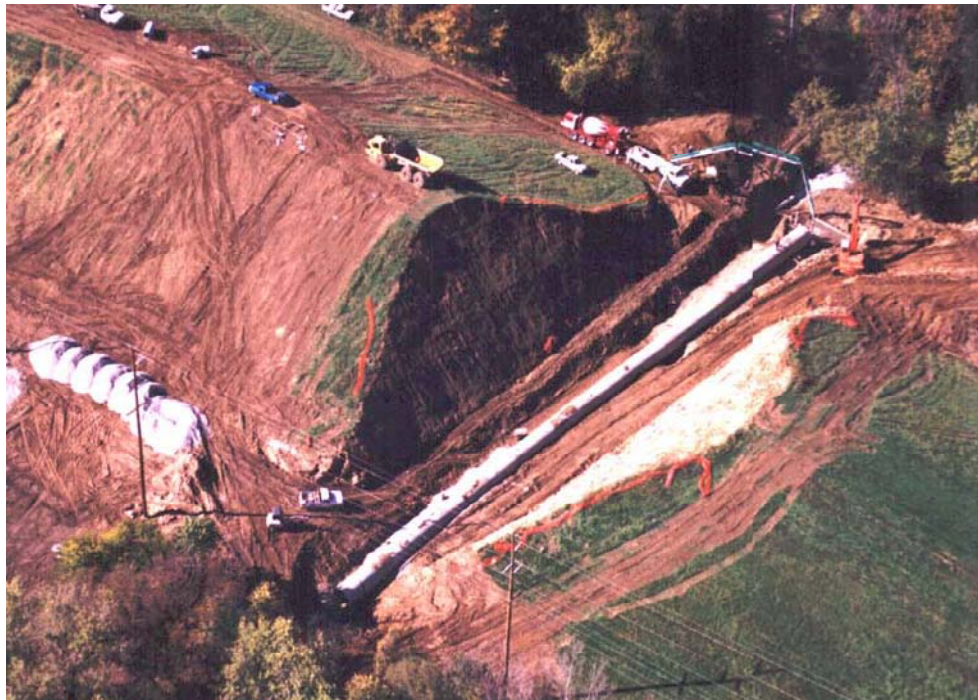
Figure A.8 –Aerial View of Replacement Procedure of an Original Levee Corrugated Metal Pipe that Had Failed and Collapsed as a Result of Corrosion. US Army Corps of Engineers
