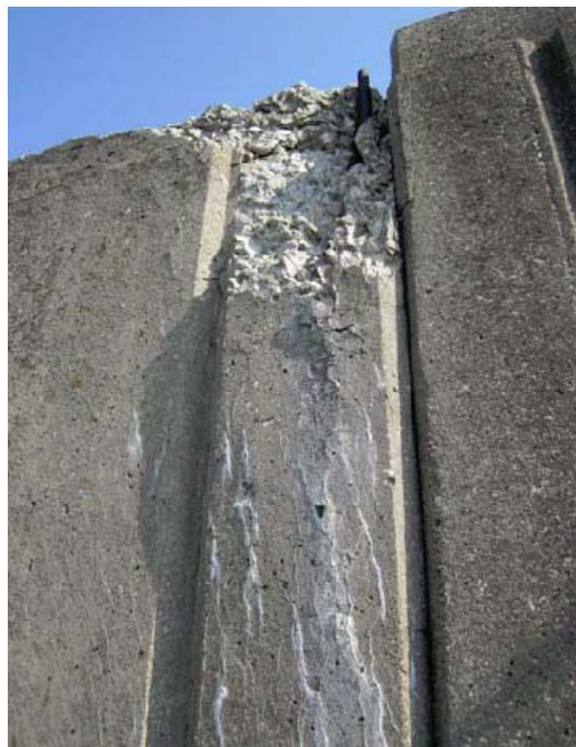
Figure A.4 – Typical Freeze-Thaw Damaged Concrete at the Top of the Newport Floodwall in Kentucky.
