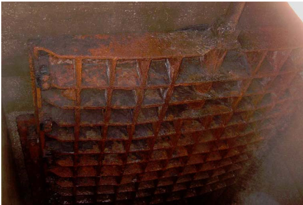
Figure A.6 – Heavily Corroded and Partially Broken 102-inch Sluice Gate in Pump Station in Paducah.
