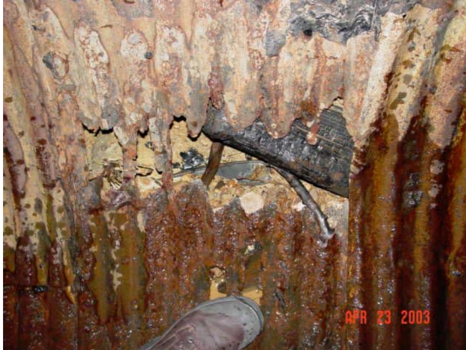
Figure A.7 – The Bottom of a Deteriorated Corrugated Metal Pipe The photo shows where the steel has been completely lost to corrosion US Army Corps of Engineers
