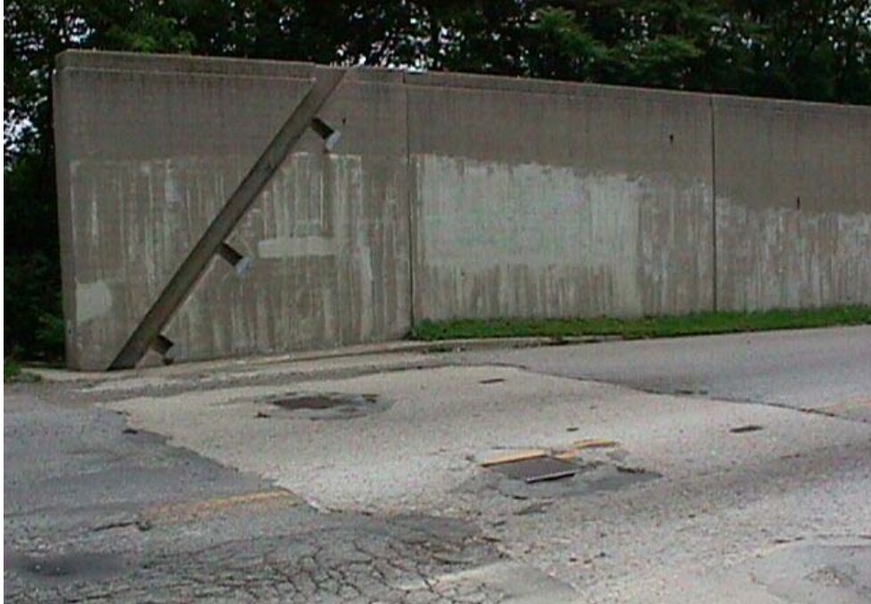
Figure A.5 – Concrete Roadway Closure Sill in Covington The sill has been damaged over time by freeze-thaw and subsequent wheel impact.
