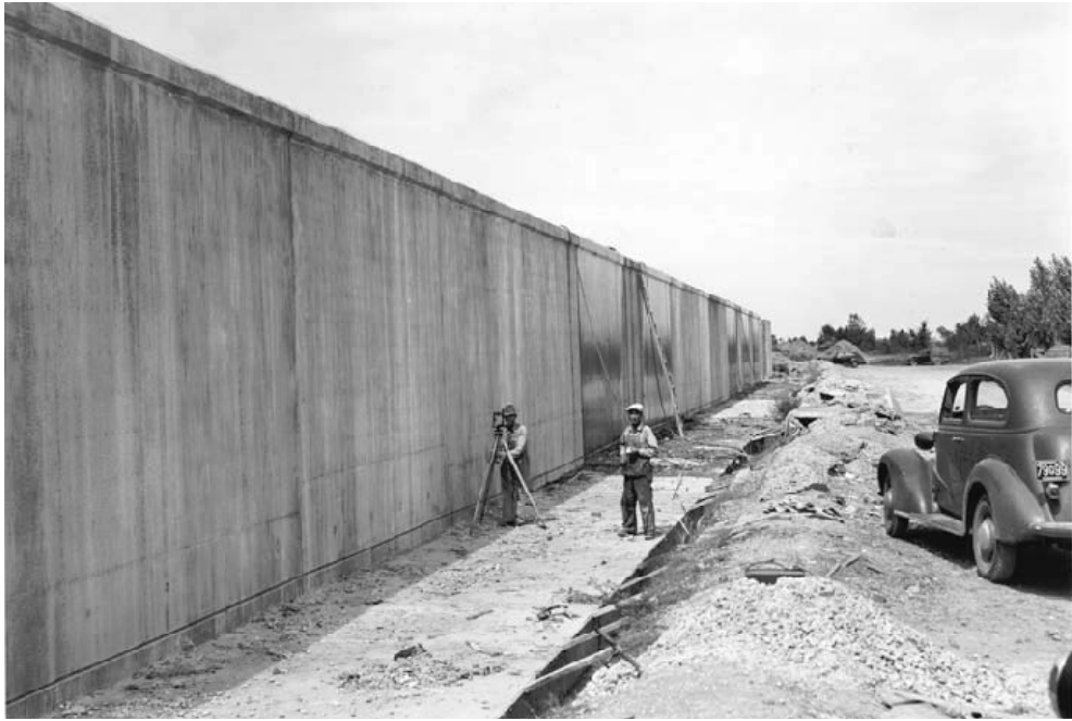
Figure A.1- Construction of the Paducah Floodwall in 1941 This Project had 15,870 lf of concrete floodwall.
